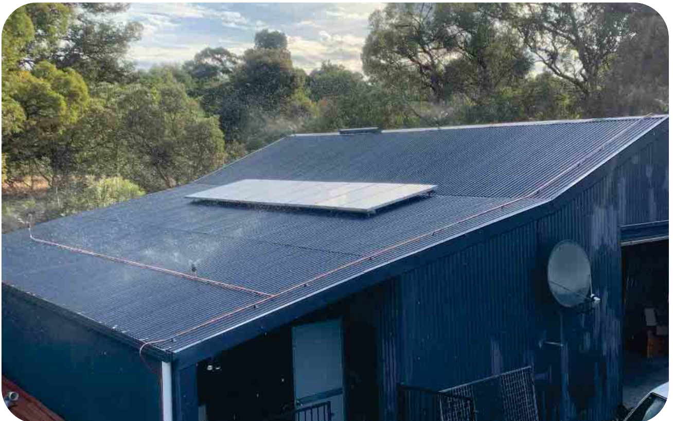
Shed roof with sprinkler set-up.
